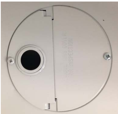
Current Junction Box
