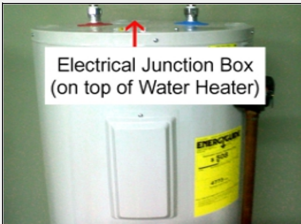
Electrical Junction Box (on top of water heater).
